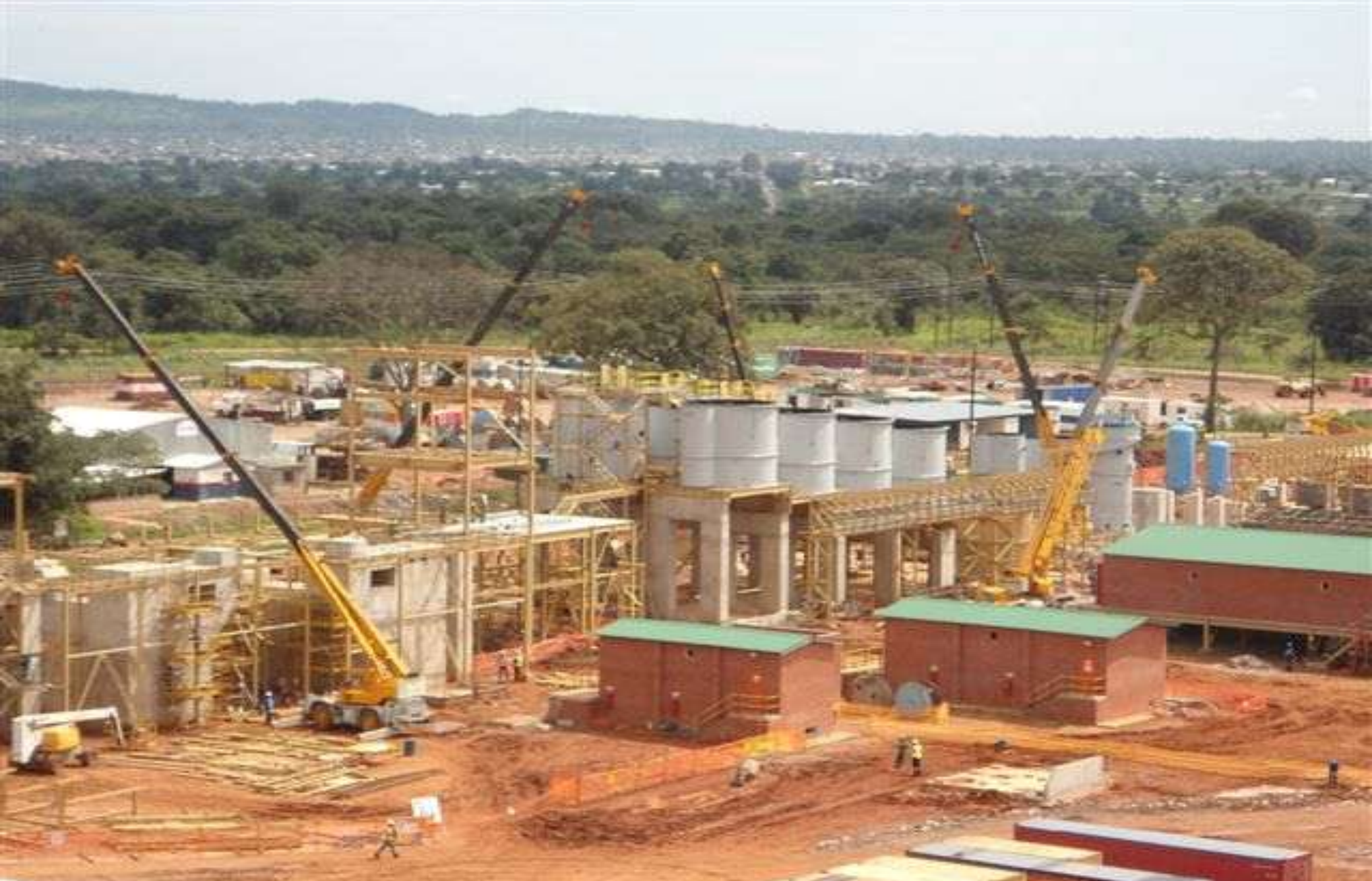
Mill and Float section at Konkola North Copper Project
